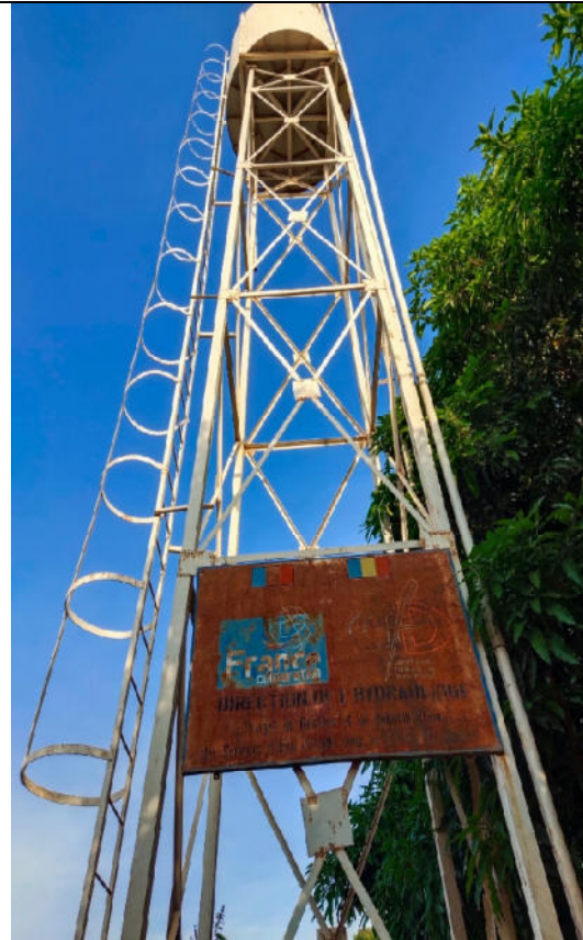
Photograph of a tube well with power pump
