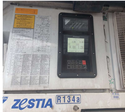
Fig 12: Control panel settings conformation
